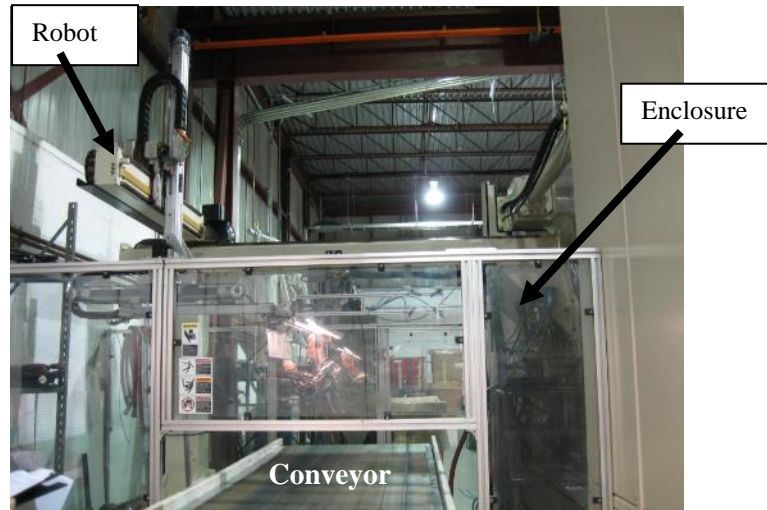
Figure 24 – Protective enclosure around the robot and the part of the conveyor with an accessible nip point.
