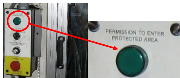
Figure 7 – Green indicator light signalling that the enclosure gate can be opened.
