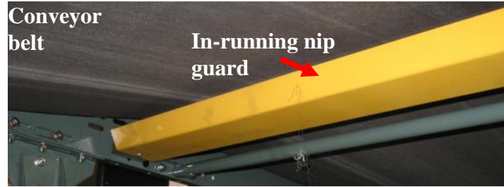
Figure 25 – In-running nip guard installed on a carrying idler of a conveyor.
