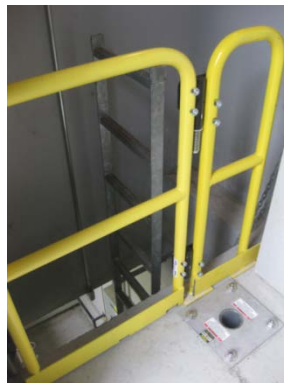
Figure 7 – Permanently installed davit arm base, ladder and railing
