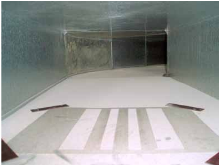
Figure 1: Return duct outfitted with sampling template
