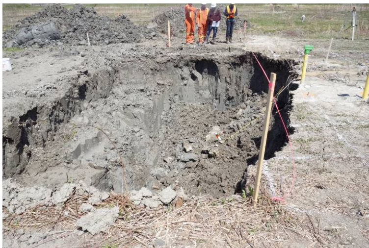
Figure 29. Rupture of vertical wall at a depth of 5 m, carrying the MPSM to bottom of the trench.
