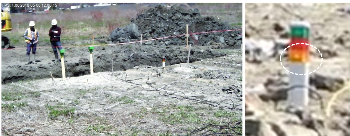
Figure 35. Flashing yellow light of D1 warning, following the detection of the second creep phenomenon prior to failure.
