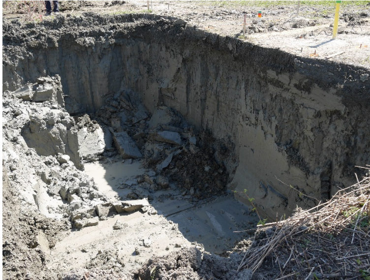
Figure 28. Rupture due to flaking and water inflow during excavation of trench A1 (step 3).
