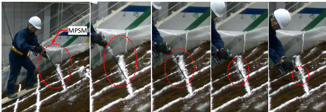
Figure 3. Installation of the MPSM by use of a hand-operated drill in less than 10 seconds.
