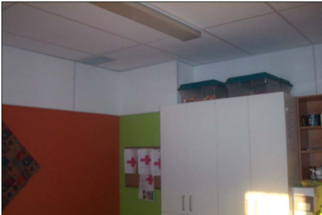
Figure 16 Acoustic ceiling with a 60 cm high band of acoustic panels installed in location A-1
